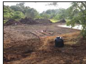
Treatment wetland which will be used as a learning laboratory for Ecological Engineering in the Tropics study abroad - Department of State grant supported - Fabio Baudrit Experiment Station, Alajuela, Costa Rica.
