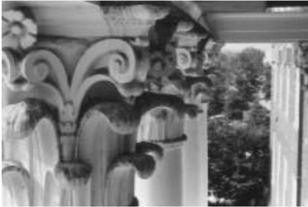
Figure 2.4. Defacement of building from pigeon droppings
