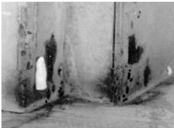
Figure 3.5. Rat droppings and grease marks
