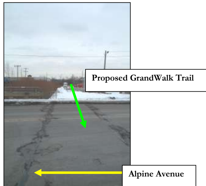
Figure 69 – Alpine Avenue intersection crossing requiring either extensive signalization or a ramped crossing
