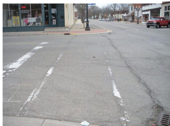
Picture 11: Worn Crosswalk Paint
