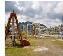
Direct-use geothermal well
