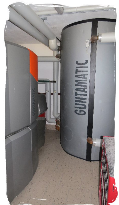
Boiler and water thermal storage tank for a chip-fed microgrid heating system.
